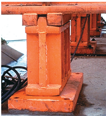
Photo 4.5 Shown is the rocker expansion bearing of a plate girder bridge. The convex surface of the rocker allows the support of the girder to move horizontally.
