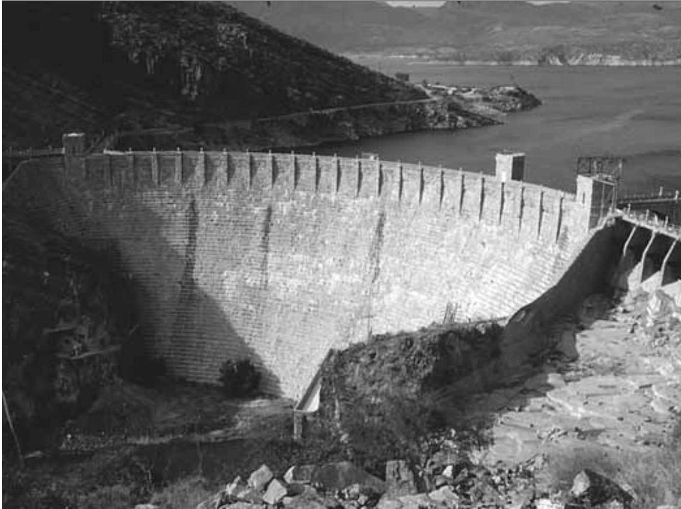
Roosevelt Dam in Arizona. Hydrostatic pressure, due to the weight of a standing fluid, can cause enormous forces and moments on large-scale structures such as a dam. Hydrostatic fluid analysis is the subject of the present chapter. (Courtesy of Dr. E.R. Degginger/Color-Pic Inc.)
