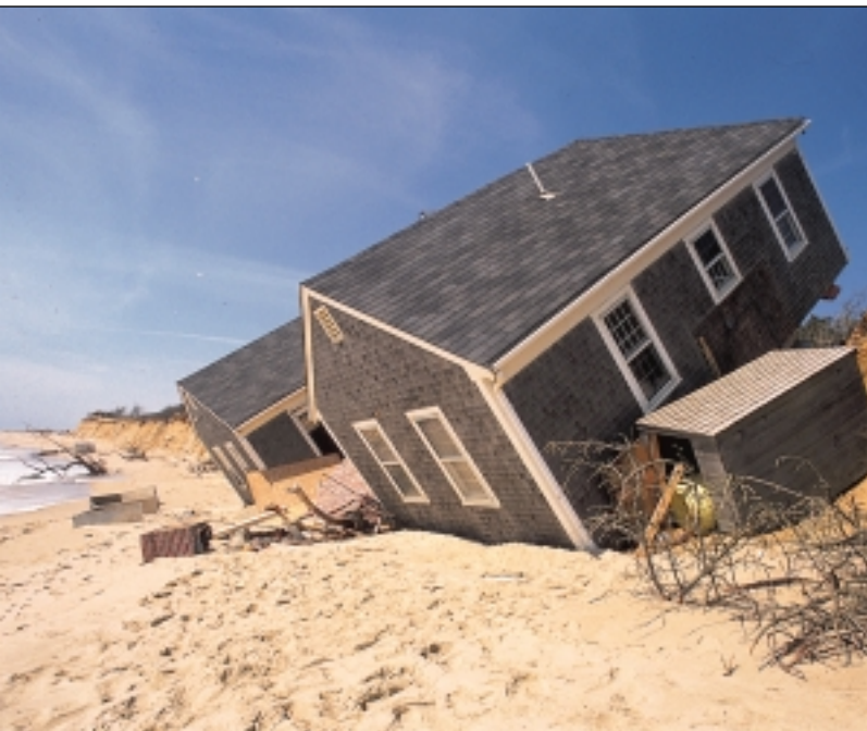
FIGURE 11.20 Winter storms have eroded the beach and undermined the foundations of homes on this barrier island. Breaking through protective dunes to build such houses damages sensitive plant communities and exposes the whole island to storm sand erosion. Coastal zone management attempts to limit development on fragile sites.
