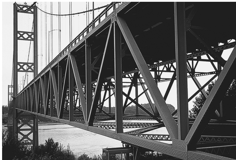
Photo 4.2: Reconstructed Tacoma Narrows bridge showing trusses used to stiffen the roadway floor system. See original bridge in Photo 2.1.
