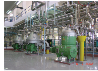
A piping network in an industrial facility
