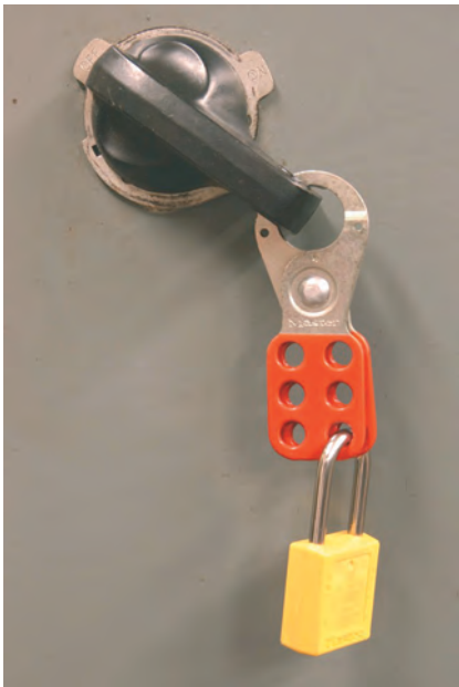
Figure 1-21 Lock it out or lock it up—never perform maintenance on a machine that can be started accidentally.
